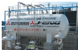
Ammonia fuel tank
