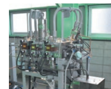
Hydrogen injection unit
