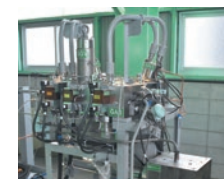
Hydrogen injection unit
