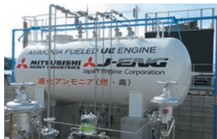
Ammonia fuel tank
