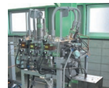
Hydrogen injection unit
